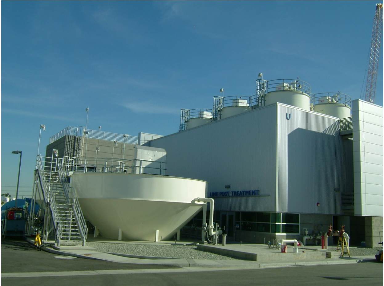
Figure 2 Lime Storage Silos and Saturator
