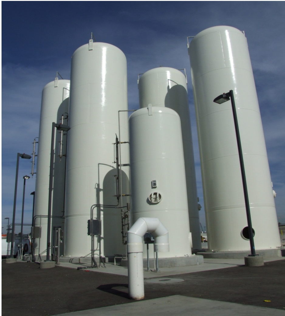
Figure 3 Carbon Dioxide Storage Tanks
