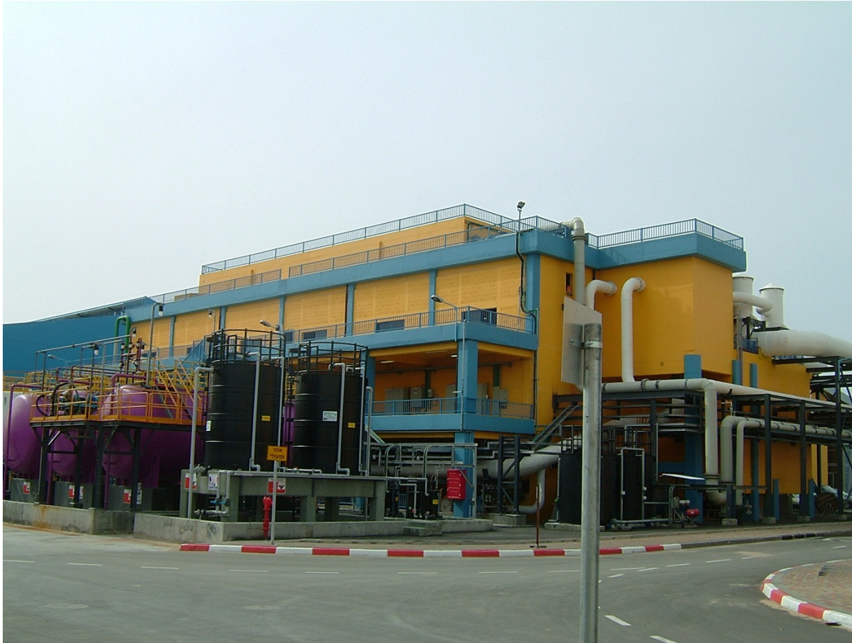
Figure 5 Calcite Contactors of Ashkelon Desalination Plant, Israel
