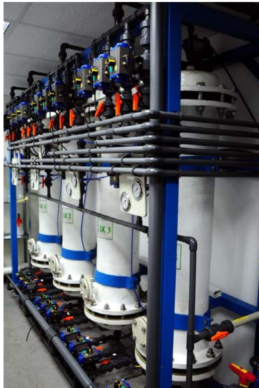
Figure 12 RWM System Ion Exchange Reactors
